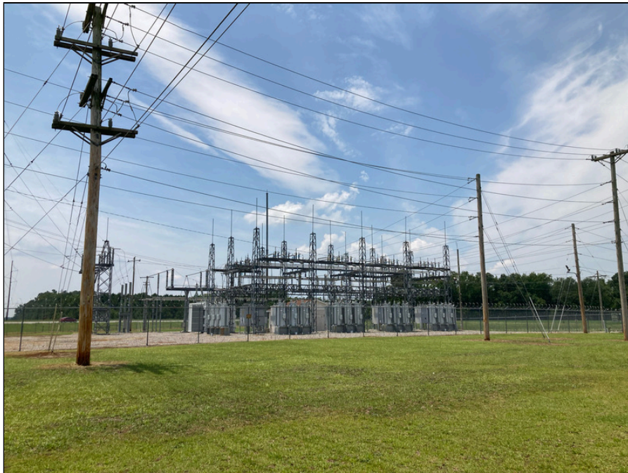
16 - View of the electrical substation on the property.
