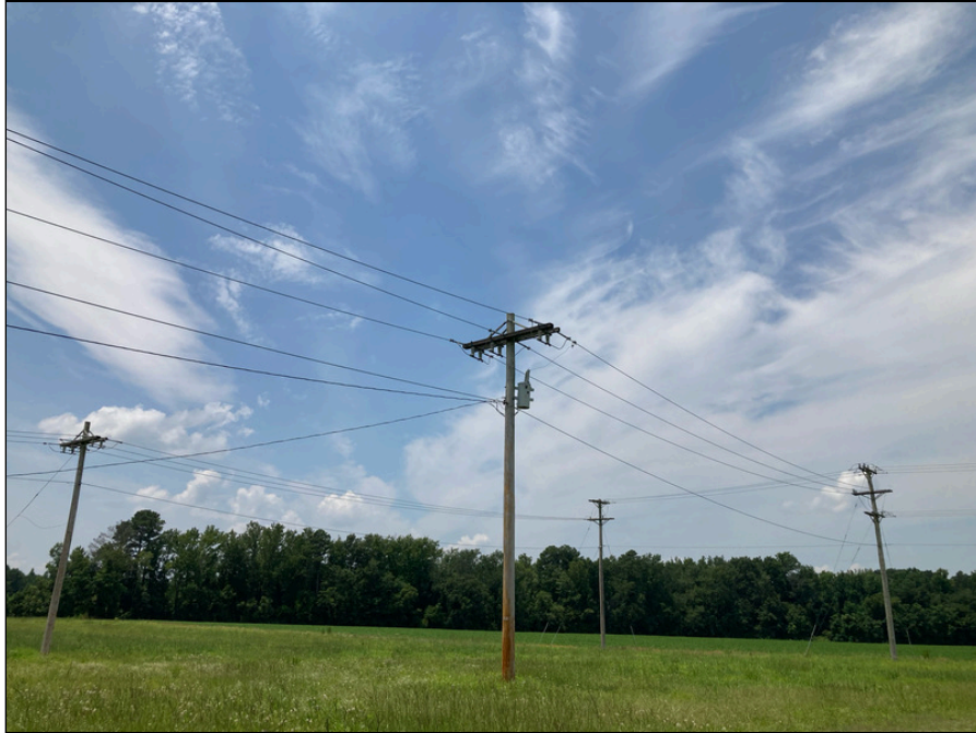
15 - View of the pole-mounted transformer on the property.
