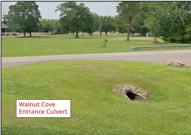
Existing Drainage System (Walnut Cove)
