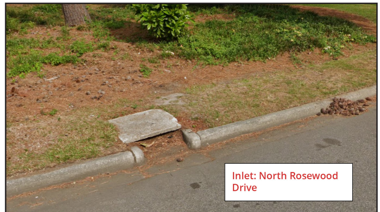
Clogged Inlet within Target Area
